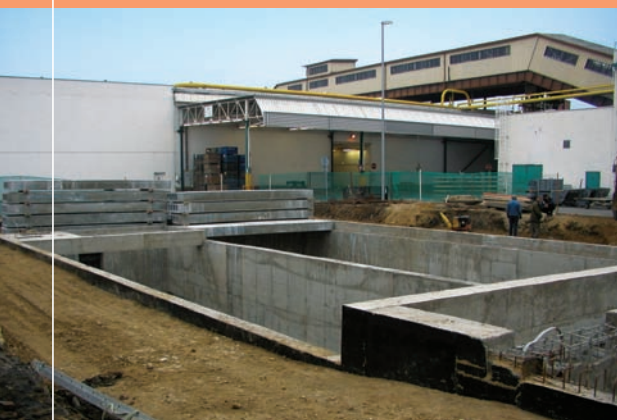
Construction of a holding tank for storm sewers in the Mladá Boleslav factory
